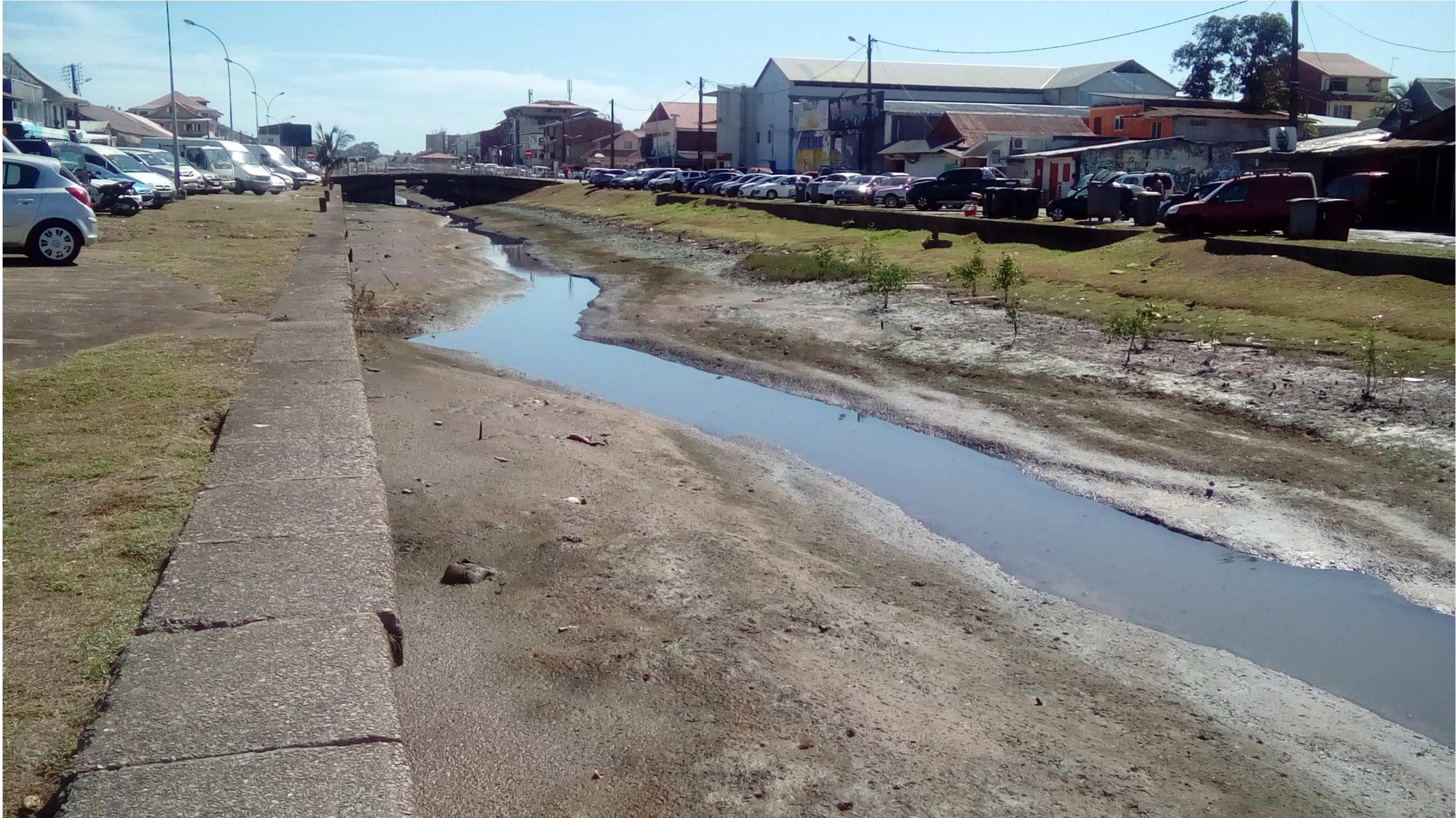
Figure 2: Photo 1 du canal Laussat
